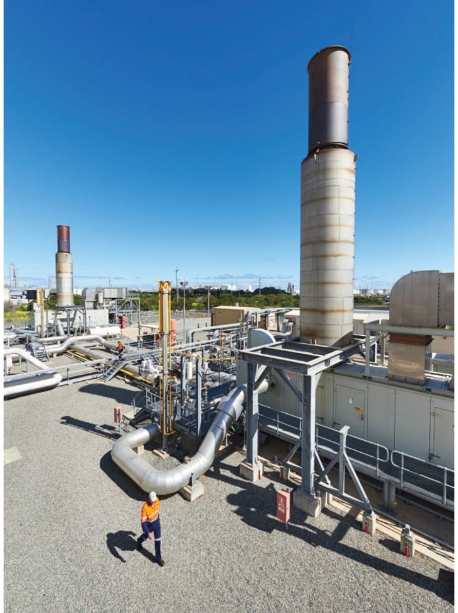
Australian Gas Networks is conducting research and running tests to bring hydrogen into their gas network, helping to decarbonise Australia's gas supply.
