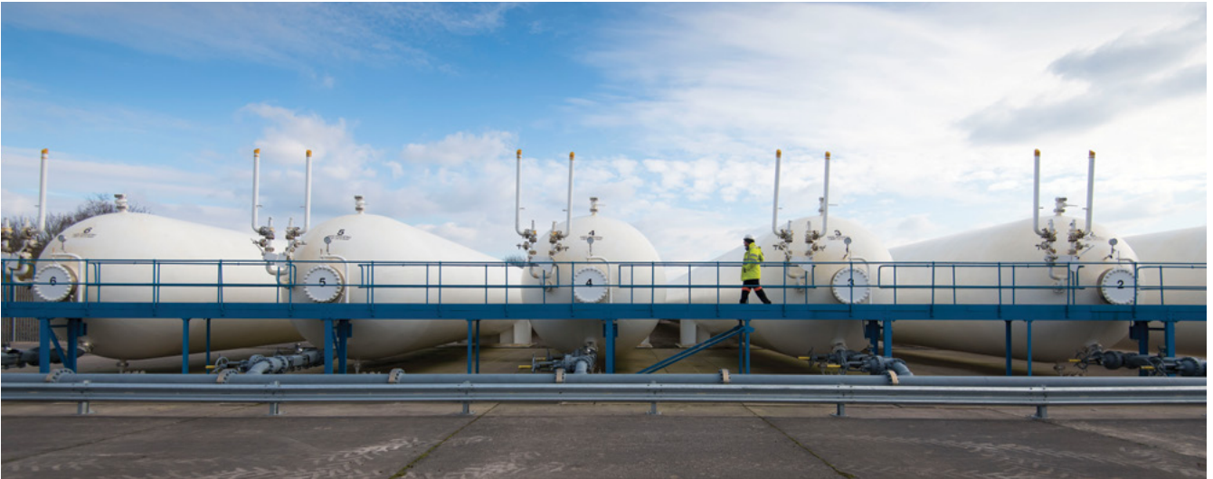
Wales & West Utilities' cylindrical steel vessels store high-pressure methane gas, contributing daily energy storage to meet heat, power and transport demands.
