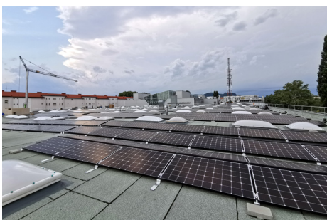
Solar panels, 3 Austria
